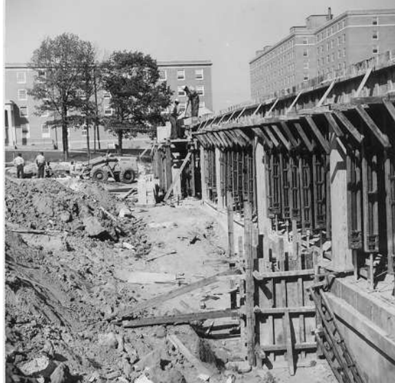
Figure 2: Initial Floor of Computer Science Center Building Construction, Centerville Hall on right, and Cambridge Hall on left, 1962, Courtesy of John Menard.
